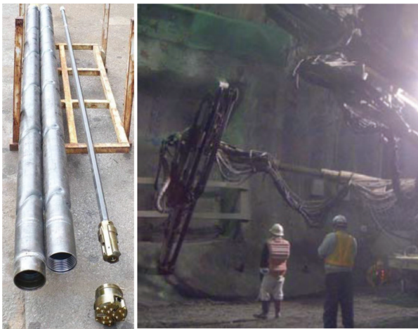
図5 段付き鋼管と掘削ビットおよび脚部補強施工状況 5) Oblique grooved pipes (right) and construction process of the foot piles
