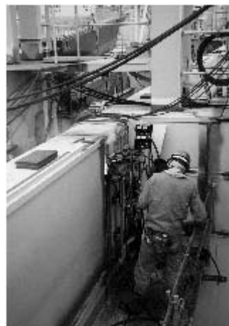
写真6 2電極VEGA ® 溶接法による溶接施工状況 An example of construction site where two-electrode VEGA ® operated
