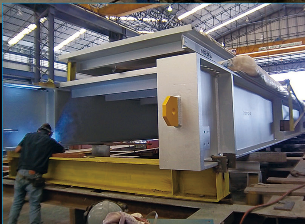
[Heat Recovery Steam Generator] Country : Thailand Product : NSHYPER BEAM™
