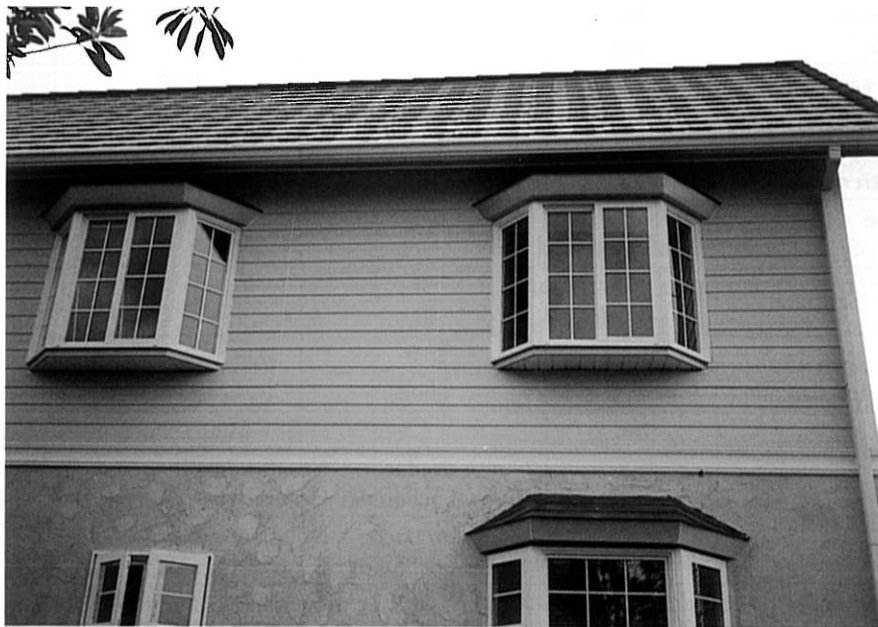
Photo 4 Moen Siding S on steel house (Moen Siding S Louver 18 mm)
