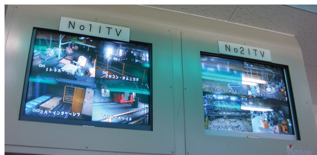
Photo 4 Monitoring screen in control room
