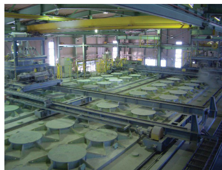
Photo 1 Raw material tanks
