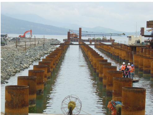
Photo 3 Driving steel pipe pile on construction of Subic Bay Port Development in Philippines
