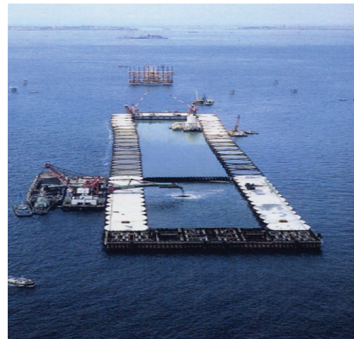
Photo 6 Revetment using straight steel sheet pile of man-made island of Tokyo Trans Bay Highway
