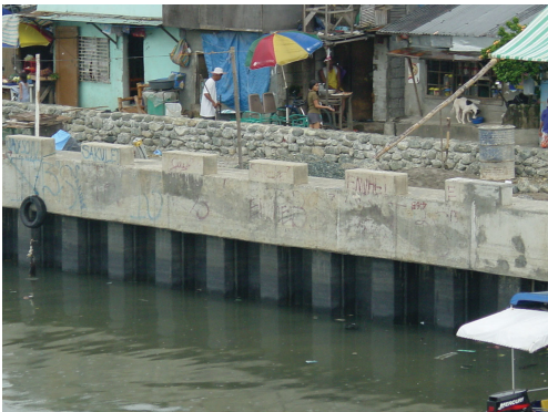
Photo 2 Revetment using 600mm wide steel sheet pile in Kamanava area of Metro Manila in Philippines
