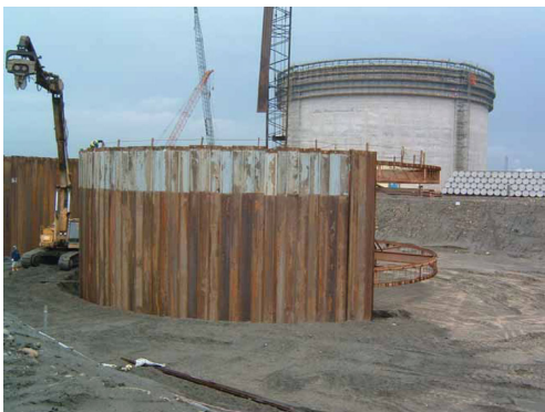
Photo 9 One by one construction method using straight steel sheet pile in Taiwan (2)
