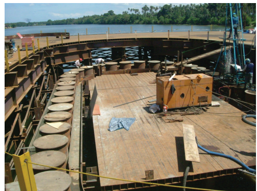
Photo 4 Construction of steel pipe sheet pile foundation for the second Magsaysay Bridge of Mindanao island in Philippines
