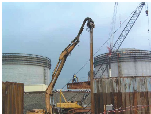
Photo 8 One by one construction method using straight steel sheet pile in Taiwan (1)
