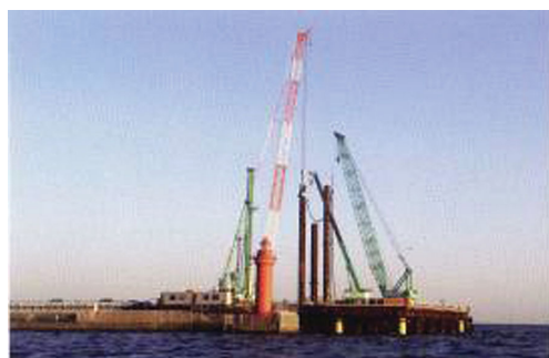
Photo 3 Pile driving on barge at the site of Tokyo Port Coastal Bridge
