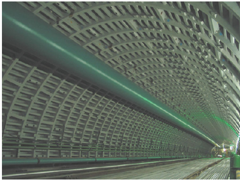
Photo 8 Large section steel segments at Tomigaya entrance tunnel of Tokyo Metropolitan Express Highway
