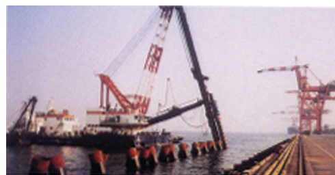
Photo 5 Pile driving by offshore pile driver at the site of Ooi container berth
