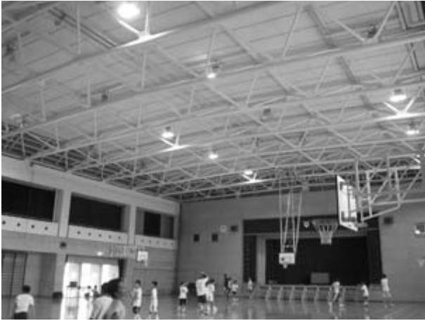
Tobata Chuo Elementary School Gymnasium, Kita-kyushu City. Designed by: Takahashi Ueda Design Corporation. Roof structure covers 24m (span) × 33m (longitudinal), and structure depth 1.2m.
