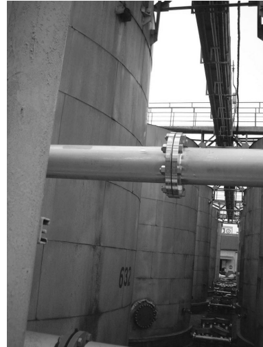
Photo 2 YUS 270 pipe with flange for a food processing plant
