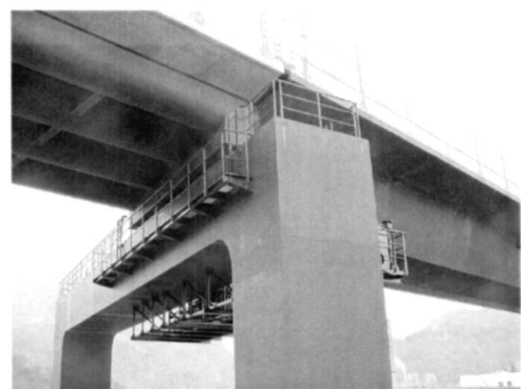
Fig. 7 A bridge for Hokuriku Bullet Train Railway over Hokuriku High Way to which 3% Ni advanced weathering steel is applied for the first time in the world, where the pipe and ship bottom like shape designs of viaducts are devised not to accumulate deposited salt, together with the application of weather resistant surface treatment called RusCor N, to realize minimum maintenance features.
