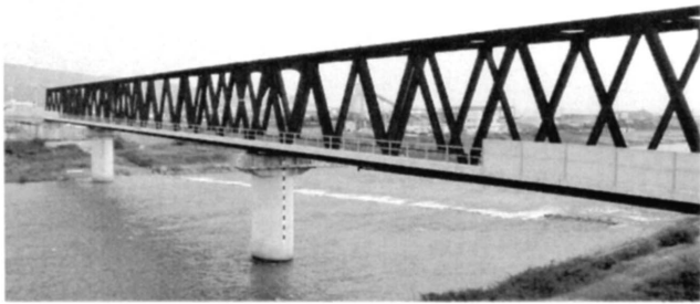
Fig. 8 Nahari Bridge for Tosa Kuroshio Railways, Kochi, Japan where 3% Ni advanced weathering steel is applied without any surface treatment.
