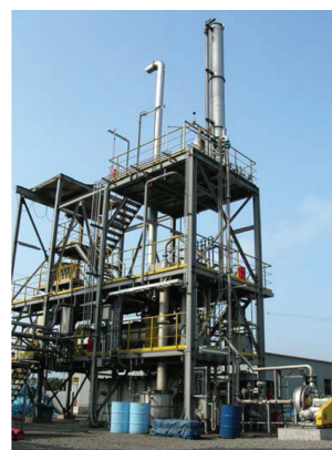
Photo 2 Appearance of PDU experimental facility
