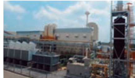
Exterior of the high-efficiency cogeneration facility
