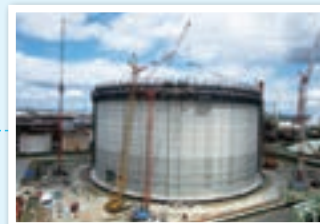
Senboku No. 1 Works No. 5 Tank of Osaka Gas Co., Ltd., currently under construction, is using 7% nickel steel sheets. With a capacity of 230,000 m 3 , this is among the world's largest LNG tanks. It will use about 3,800 tons of steel sheets.
