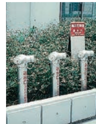
連結送水管 Connecting Water Supplying Pipe
