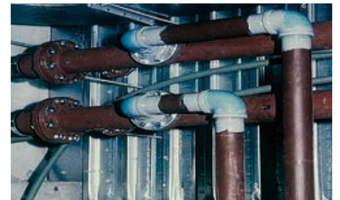
屋内給水配管 Water Supply Pipe Line
