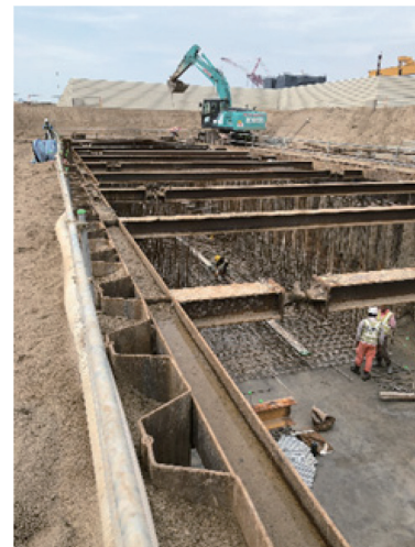
Fig. 1 Application of HAT-type steel sheet pile on temporary retaining wall in Singapore
