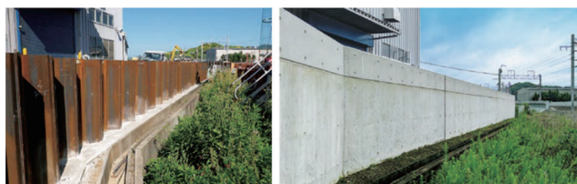
Fig. 3 Steel barrier wall for flood control: under construction (left) and completion (right) 6)
