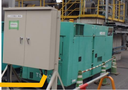
[Emergency power generator]
