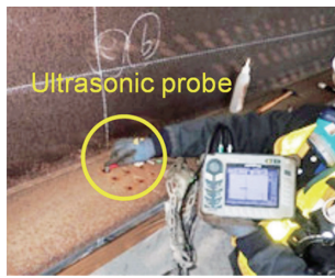
図2 現場での超音波による板厚測定写真 On-site thickness measurement of steel plate by ultrasonic equipment
