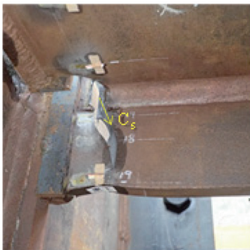
(c) No. 5 : Flange fracture at beam-end weld hole
