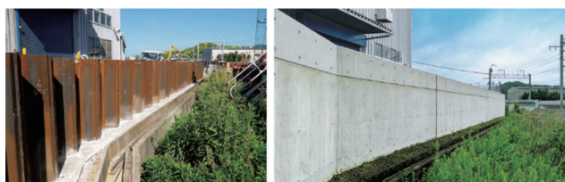
図3 浸水対策用鋼製遮水壁の施工中（左）と施工後（右） 6) Steel barrier wall for flood control: under construction (left) and completion (right) 6)
