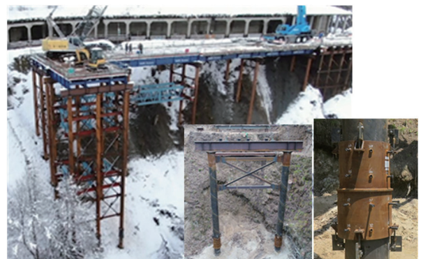
図3 鋼管杭を用いた構造例と継手構造 Example of structure using steel pipe piles and lateral connection
